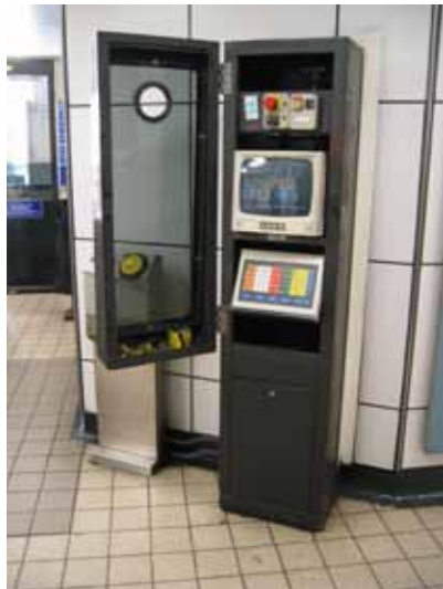
Typical Ticket Hall Station Control Unit
