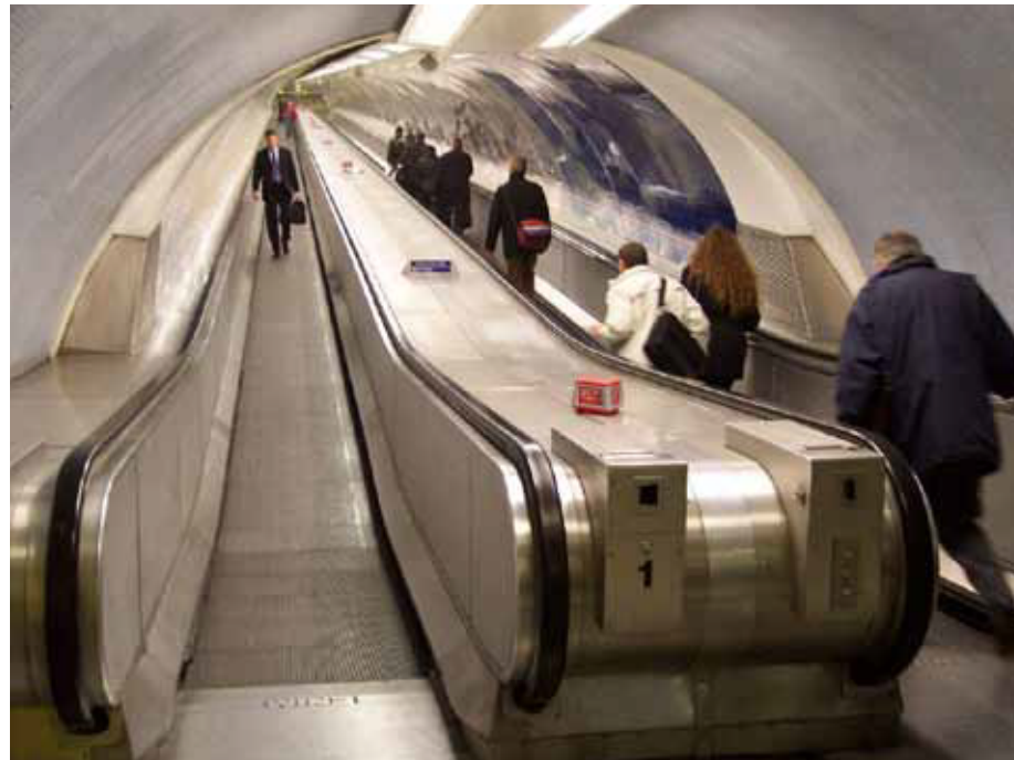
Typical passenger conveyor
